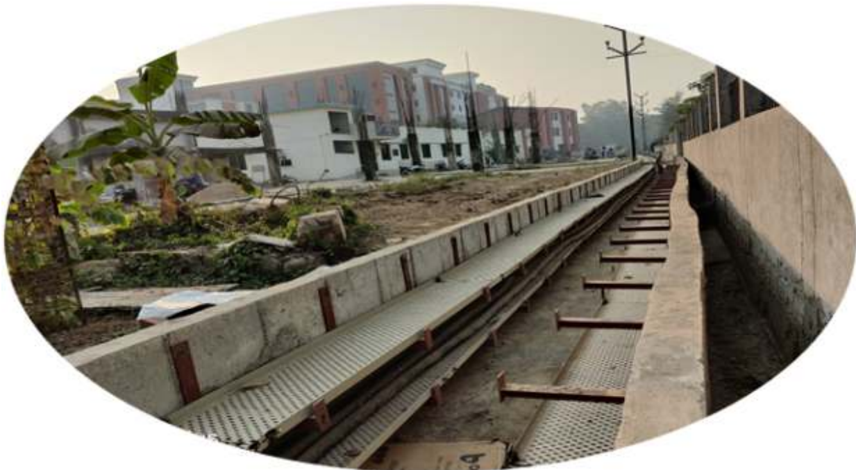
Cable trench from 33KV Sub Station to 11KV old sub-station and 11 KV new Sub-station
